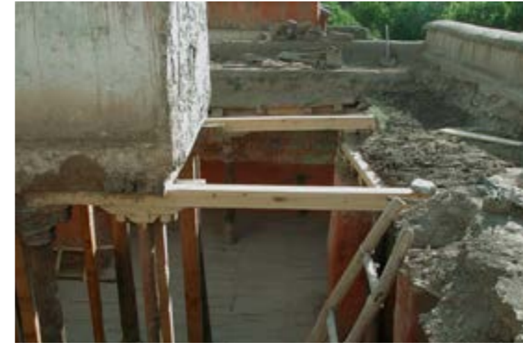
485 Restoration of the courtyard in 2003. A careful look at this image reveals that excessive height of clay used for the courtyard's roof and the disintegrated plastic sheets within it. CL 2003 (9564).
